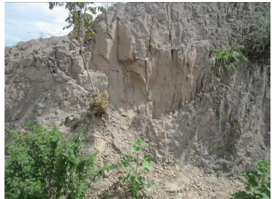
Figure 4 Deformation and fracture on the south slope side
